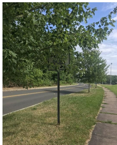
Photograph 4. Trees which obscure important traffic signs should be pruned to improve visibility. In this instance, the sign being obscured is a parking sign, which could potentially be moved to avoid the need for repeated pruning of the tree.
