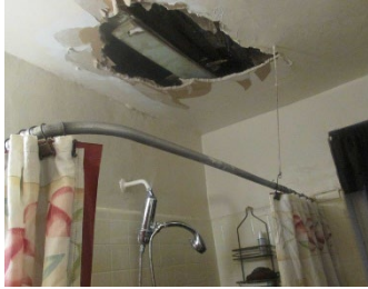
Holes in Walls/Ceiling
